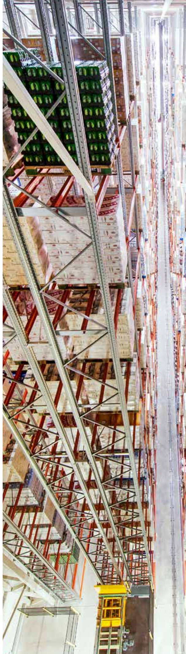
Crane racking | 10,000 pallet positions
